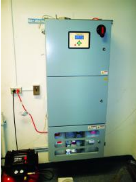
A THM analyzer was installed to monitor the THM levels of the incoming water from Middlesex Water Co. as well as the THM levels of the water leaving the tank.
